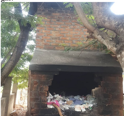
Figure 1a: Broken burning structure
