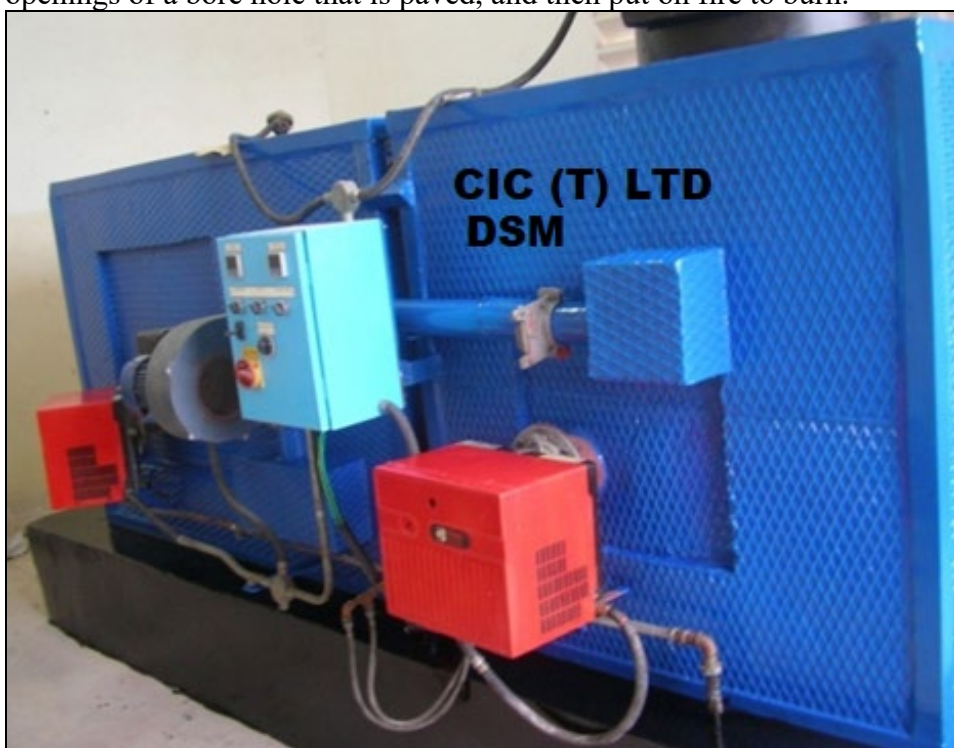
Figure 2: High-Tech incinerator at Temeke Referral Regional Hospital
